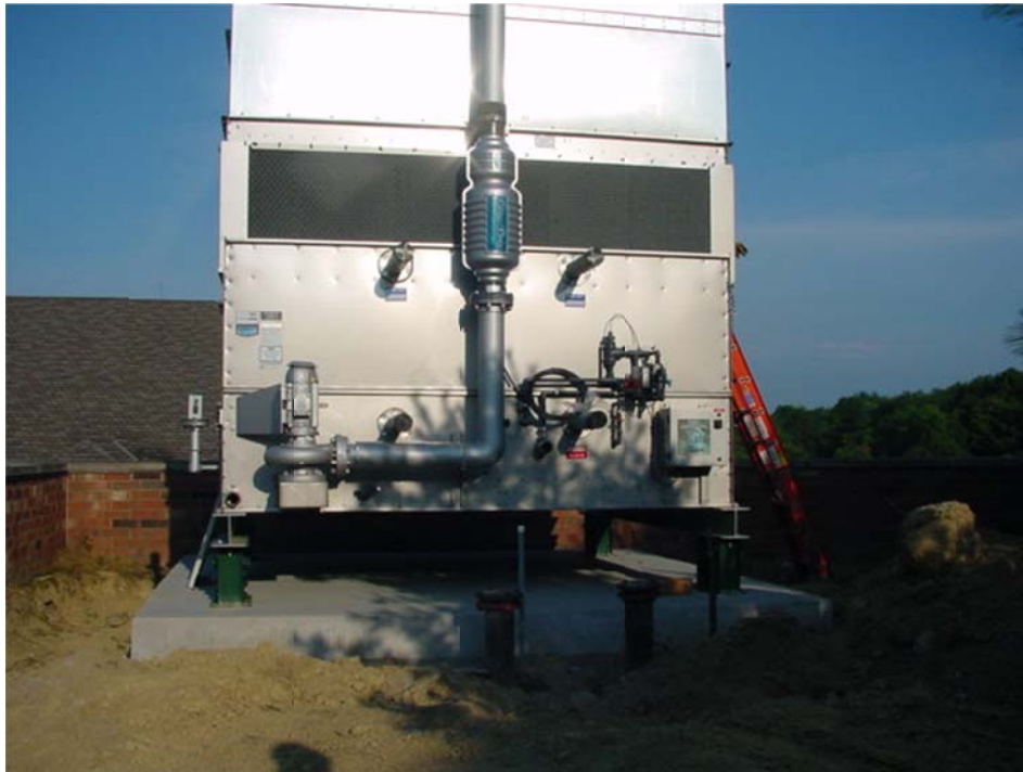
(Figure 4: Cooling Tower)
